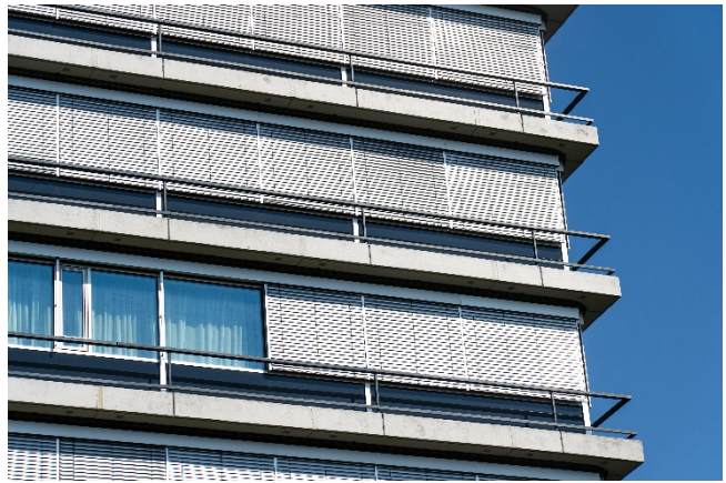
Image 2: The building is particularly worthy of preservation thanks to its curtain wall with all-round balconies. One special feature are the narrow aluminium profiles that give the façade its structure. (Source: HUECK)
